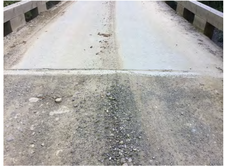
Minor damage noted to top of ballast wall and panel 1 at right bank
